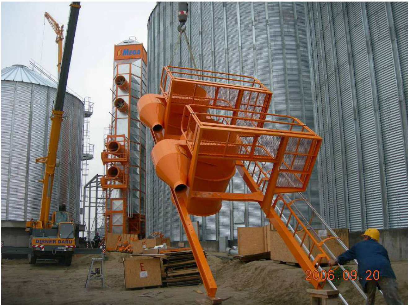
Separadores de Polvo durante montaje. Dust and Fine Collector system during the assembly process.
